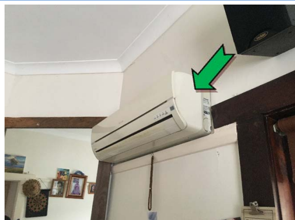
Photo 12. Interior, living room, air conditioning unit – non ODS-containing refrigerant gas.
