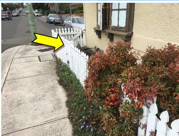
Photo 11. Exterior, throughout, fence – suspected lead-containing white upper paint systems.
