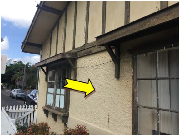
Photo 9. Exterior, throughout, walls – suspected lead-containing cream upper paint systems.
