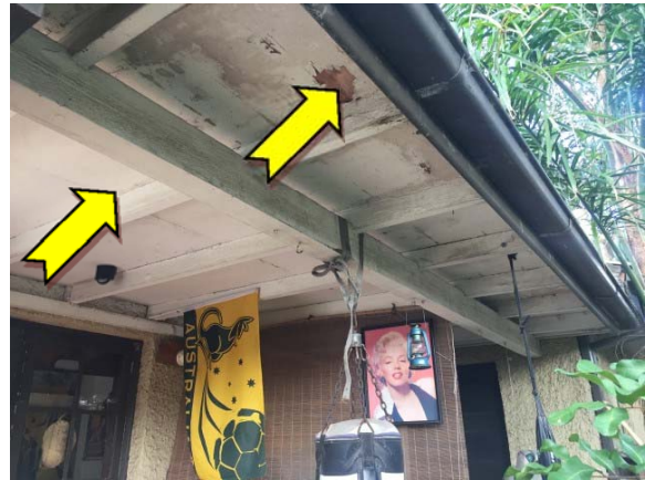
Photo 10. Exterior, throughout, north-east awning – suspected lead-containing white upper and pink lower coloured paint systems.
