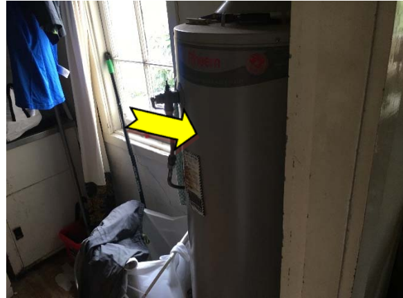
Photo 8. Interior, washroom, hot water heater – suspected SMF internal insulation material.
