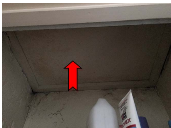
Photo 6. Interior, cupboard, infill panel to form ceiling – suspected asbestos-containing fibre cement sheeting.
