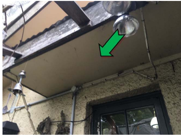
Photo 4. Exterior, rec room, new extension, north, south and west elevation, eaves – non asbestos-containing fibre cement sheeting.
