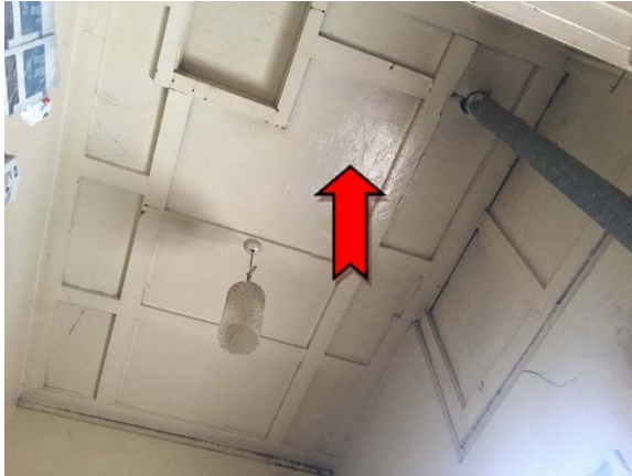
Photo 7. Interior, washroom, ceiling – suspected asbestos-containing fibre cement sheeting.
